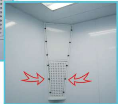
filter for outlet, removes gas to keep the environment safe
