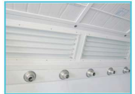
Water painting compliant
