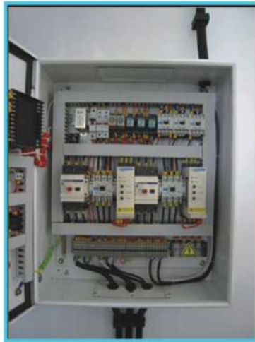
High quality electric components and precise installation
